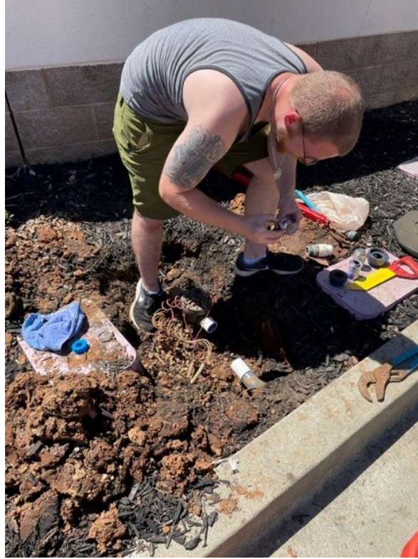
Facility Maintenance Worker Ashton repairs an irrigation water main at the Community Center.
